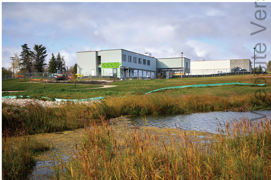
Construction of the treatment centre along the banks of the Sturgeon Creek October 2020. Photo: Ian McCausland
