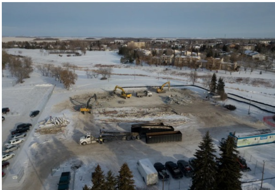
Demolition of Vimy Arena to construct the treatment centre, Dec 2019. Photo: Storm The Castle Media
