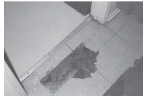
Excessively worn flooring is unsightly and contributes to sub-floor damage.
