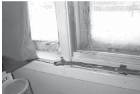
Windows that need replacing can cause frost, condensation and mould.
