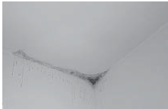
Moisture related damage and mould at ceiling can be caused by poor ventilation and/or insulation.
